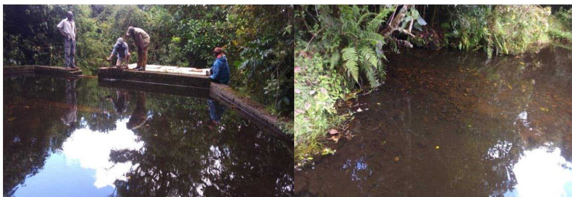
The Intake where we need construct the aluminum strainer and placement of some water filters
