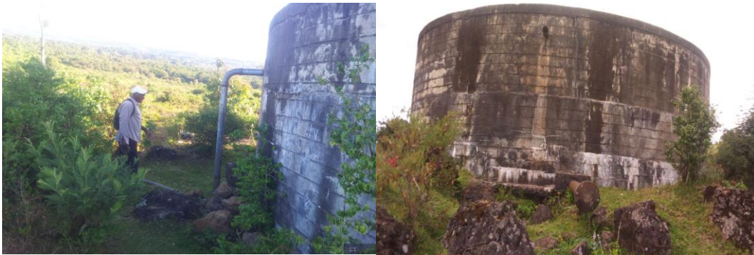
LOWASA project 100,000 liters' masonry tank from its inlet to washout., where the propose rehabilitation phase 1 will end while waiting for phase 2 which include Building 3 break pressure tanks of 20 m 3 each
